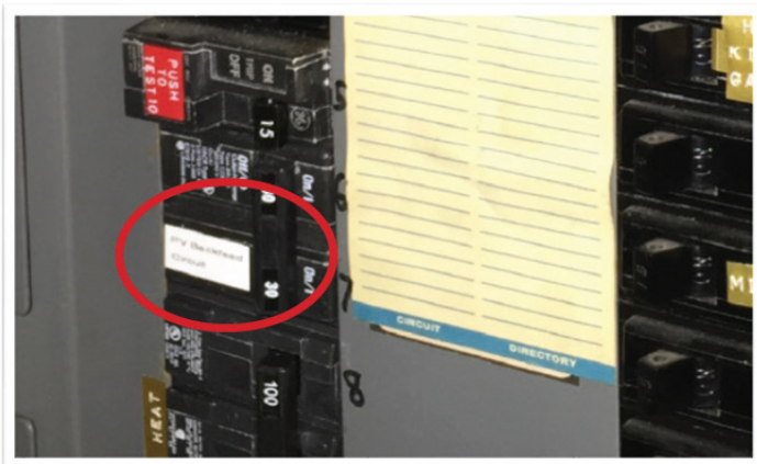
Photo 3: Working clearance not maintained: NEC 110.26
