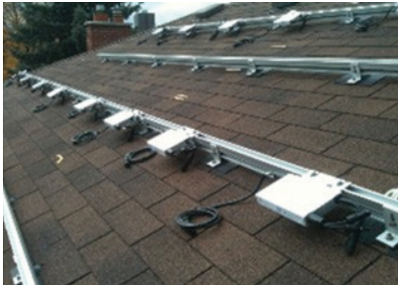
A Solar Electric Racking System
