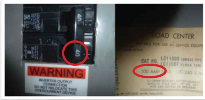
Photo 2: Backfed PV breaker not installed at opposite end of buss bar from main breaker: 2014 NEC690.12(D)(2)(3)(b)
