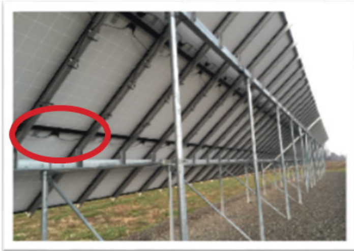
Photo 5 - Conductors over 30V not guarded, installed in raceway, or otherwise inaccessible: NEC 690.31(A)
